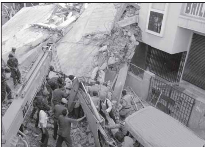
The collapsed 5- storied building under construction on Narayanguda Main Road
